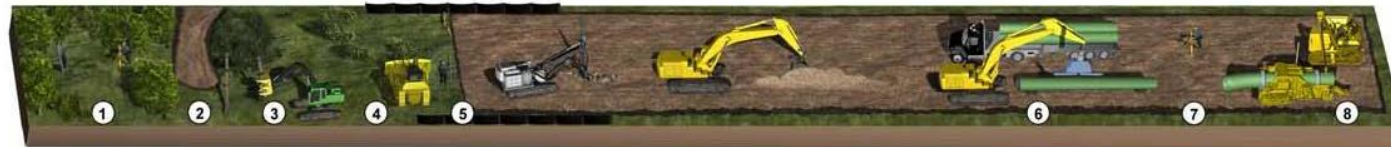
1. Survey and Staking 2. Access Road Development 3. Clearing* 4. Installation of Sedimentation and Erosion Controls 5. Grading 6. Stringing 7. Engineering Bends 8. Pipe Bending Bends
